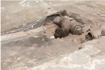
Old plumbing line was exposed with a deep floor cavity.
