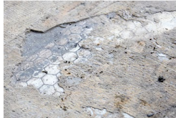
The deteriorating subfloor covered in old glue was exposing some of the original ceramic tiles.
